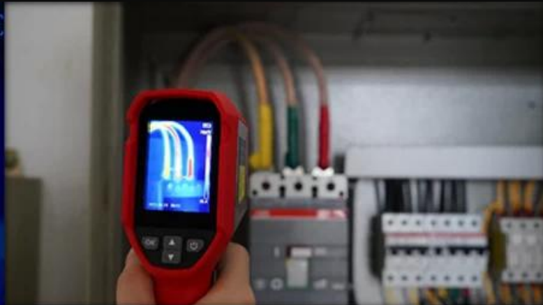
Inspection of Distribution Cabinet
